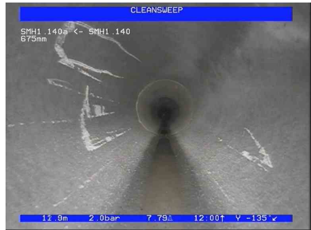
2, 00:01:26, 11.90 m General remark, Scrape damage visible
